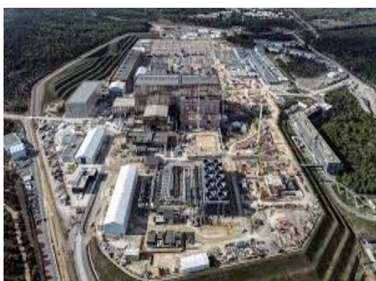
©ITER – The site
