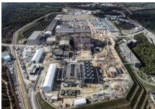
©ITER – The site
